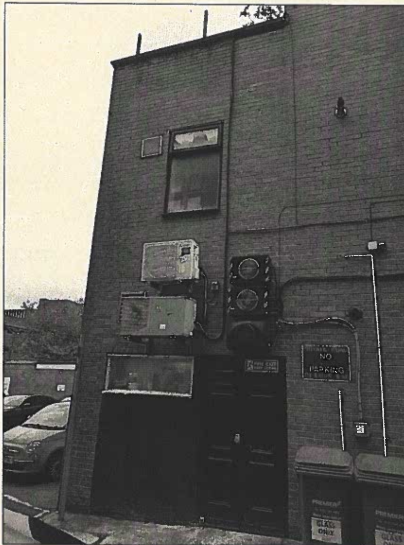
Figure 4: External Plant of 'Sky Sports Bar'
